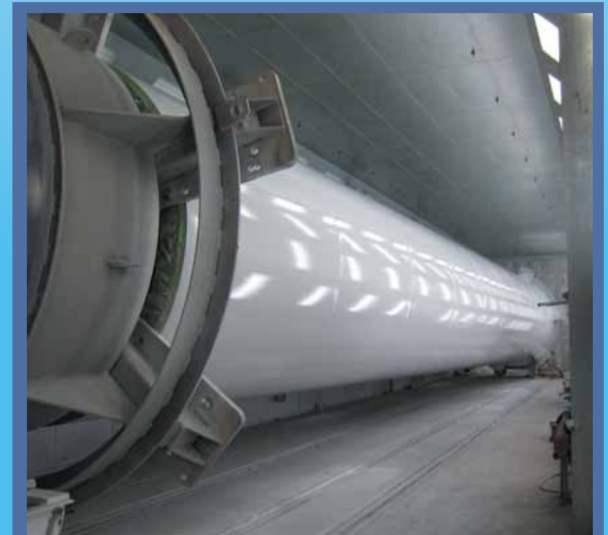
Ameron Paint Booth No. 3. Finish Coated Upper Section to 80 meter tower- Booth #3
