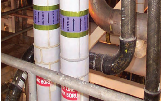
Bondstrand cooling water lines in service
