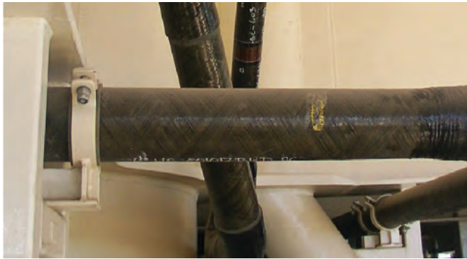
Crossing of Several Pipe Systems
