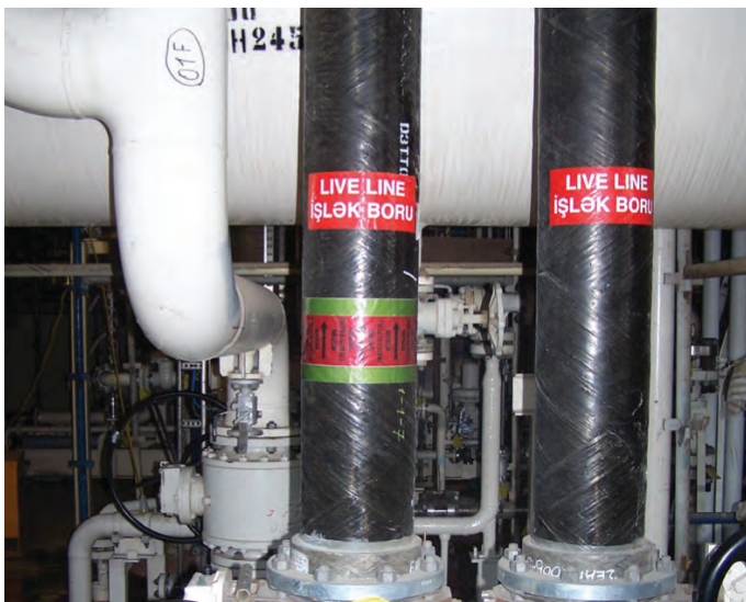
Flanges to connect to steel piping
