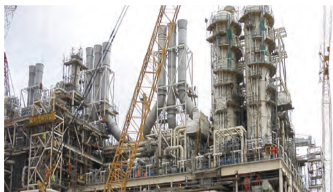
C&WP platform in production
