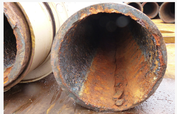
Corroded chrome-iron alloy piping removed from service
