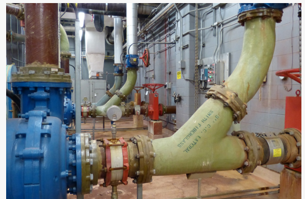
Ash Pump Piping
