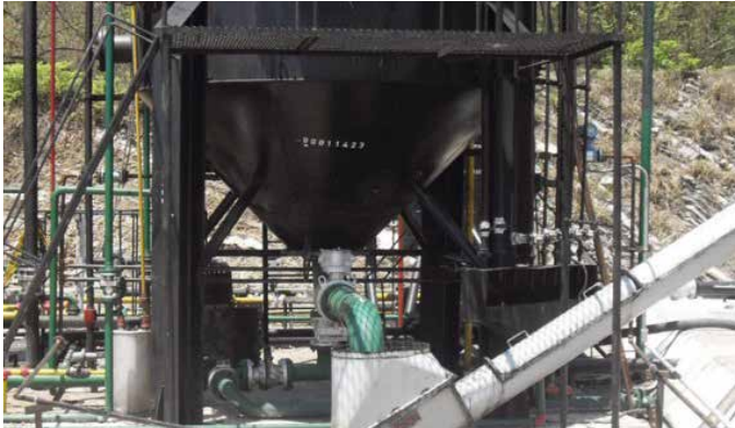
Figure: Heater-treater conical bottom with screw conveyor.
