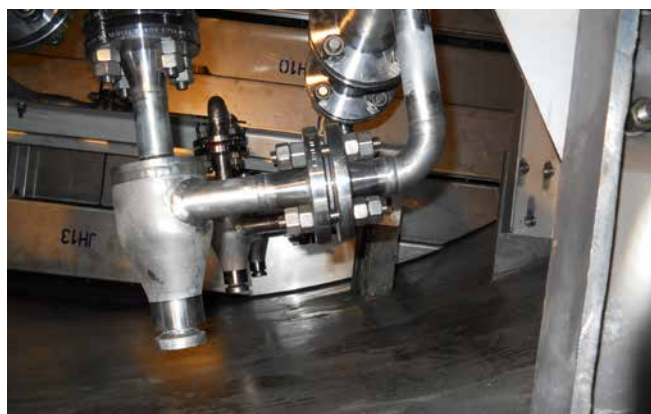
Figure: ToreOVD installed in a separator for connection to a ToreScrub
