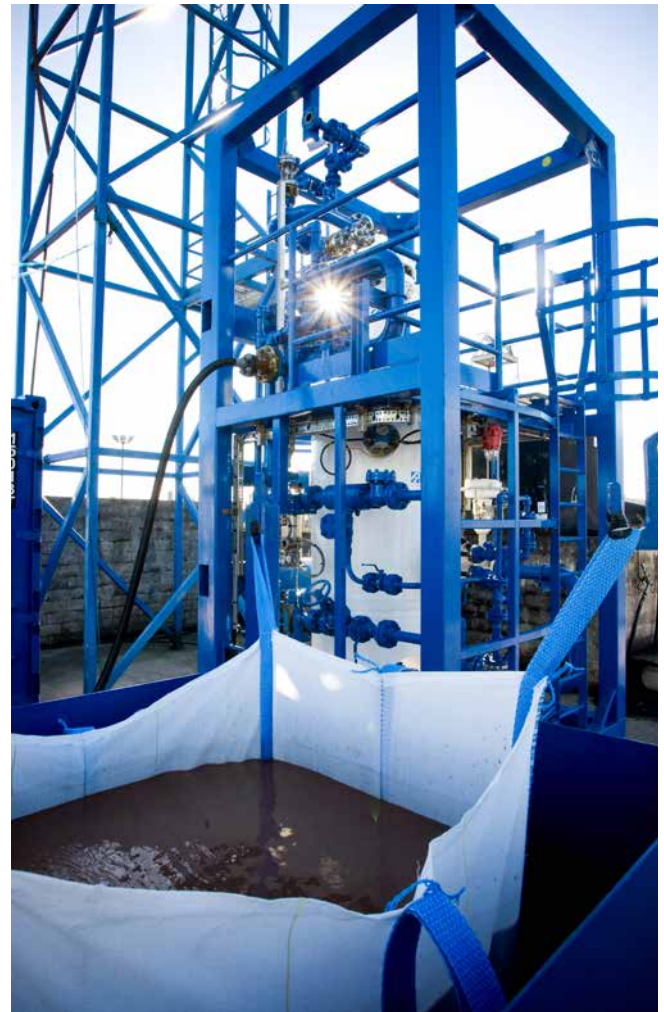
Figure: NOV ToreScrub rental unit for temporary vessel desanding
