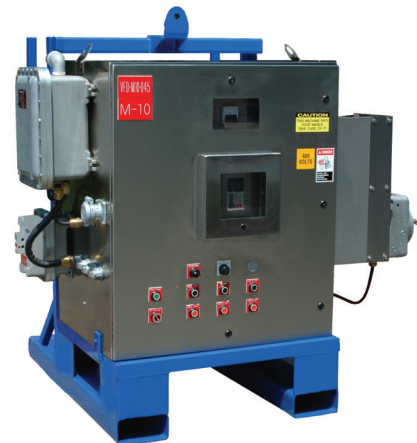
Panel controlador VFD
