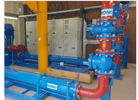
Sewage pumps and MCC
