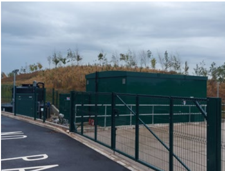
Pump station exterior
