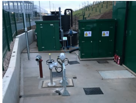
Dosing plant, Mains Incomer and Actuated Valves.
